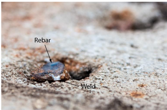
Figure 3 – Typical Weld Failure
