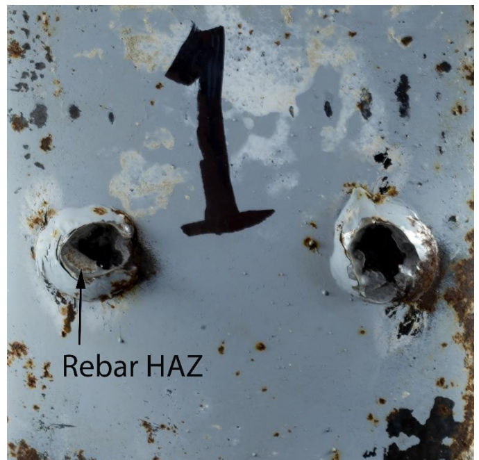
Figure 4 – Failed Weld Joint on Bracket
